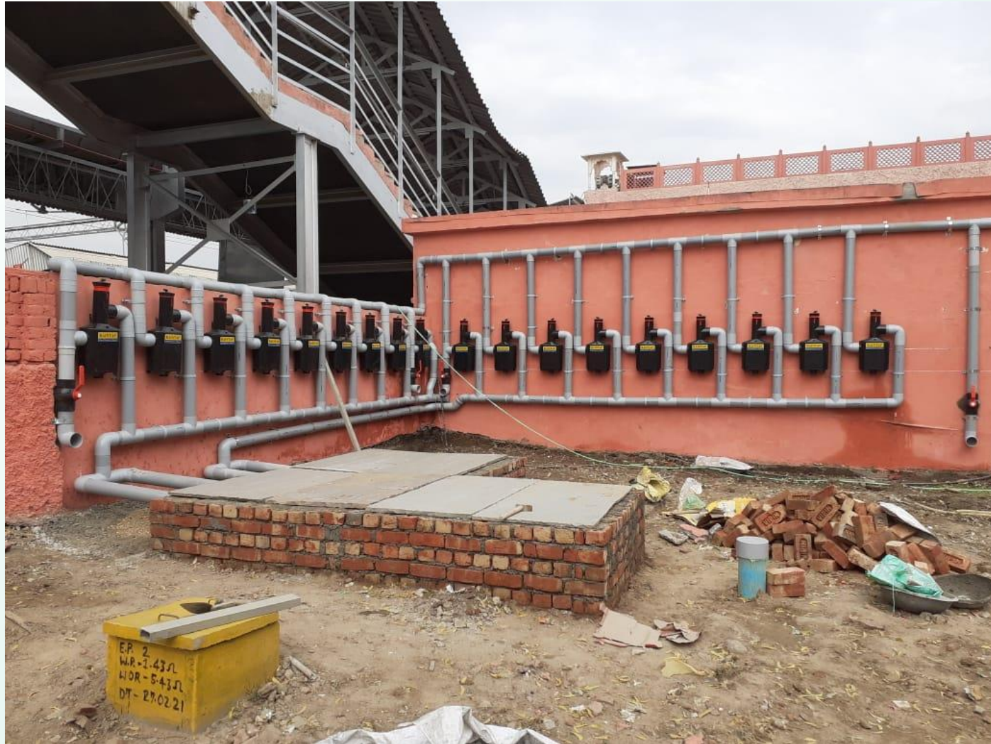
Rainwater Recharge at Railway Station
