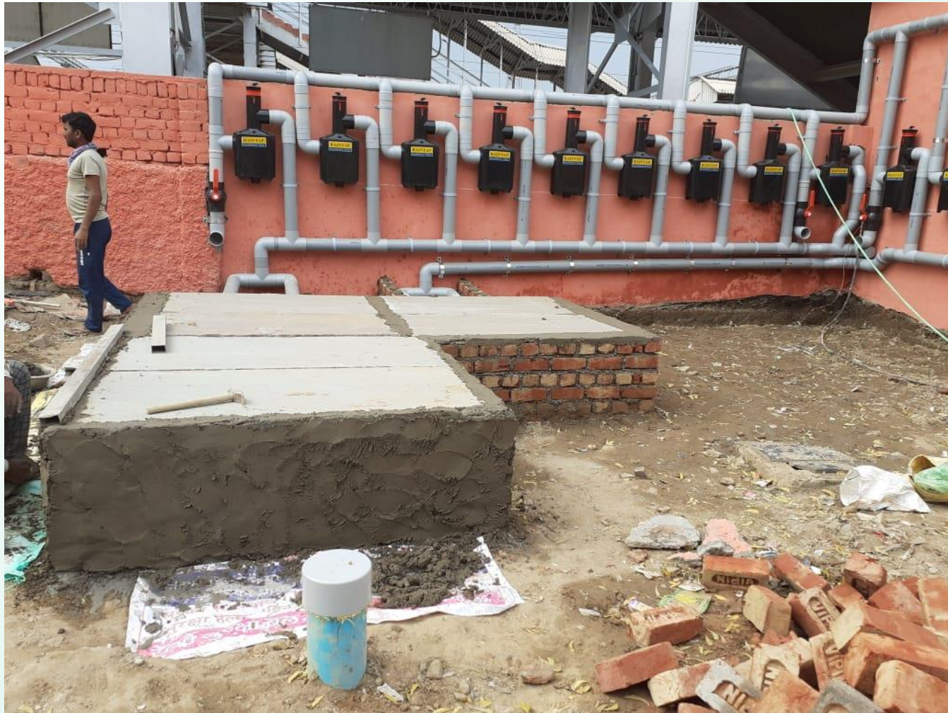
Rainwater Recharge at Railway Station
